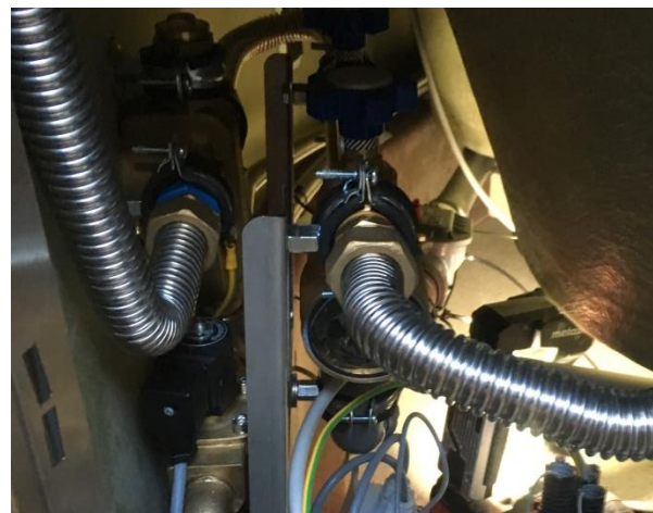
Figure 3 Water connection pool side.
